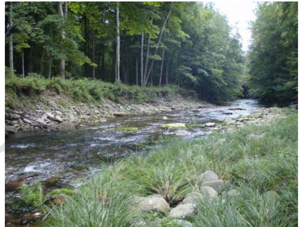
Figure 5 Bank erosion, Stn 25700, left
