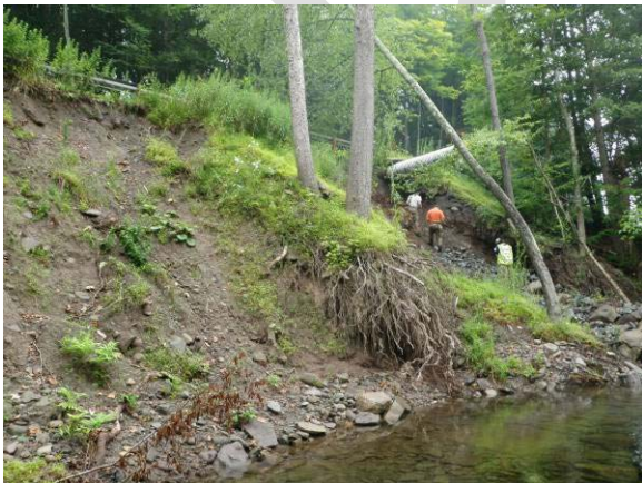
Figure 9 Eroding embankment along SC Rte 153
