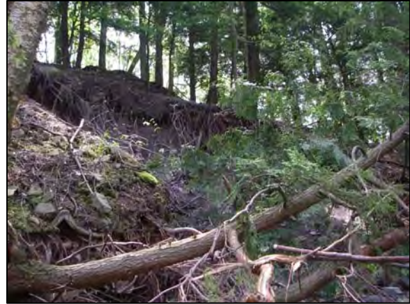
Bank erosion at Station 62100
