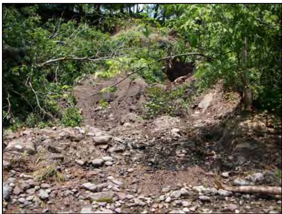
Bank erosion at Station 45560
