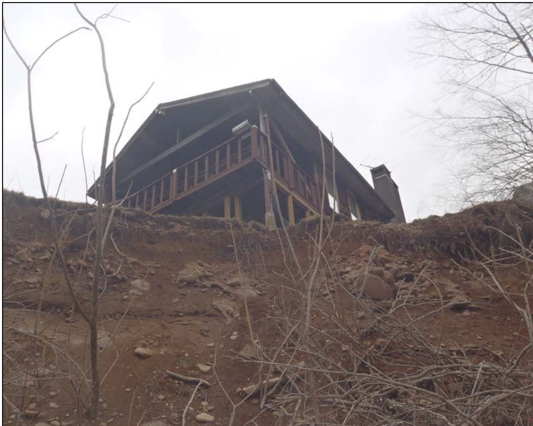
Figure 7. Residential structure in the Town of Hunter hanging over a failed streamside hillslope.
