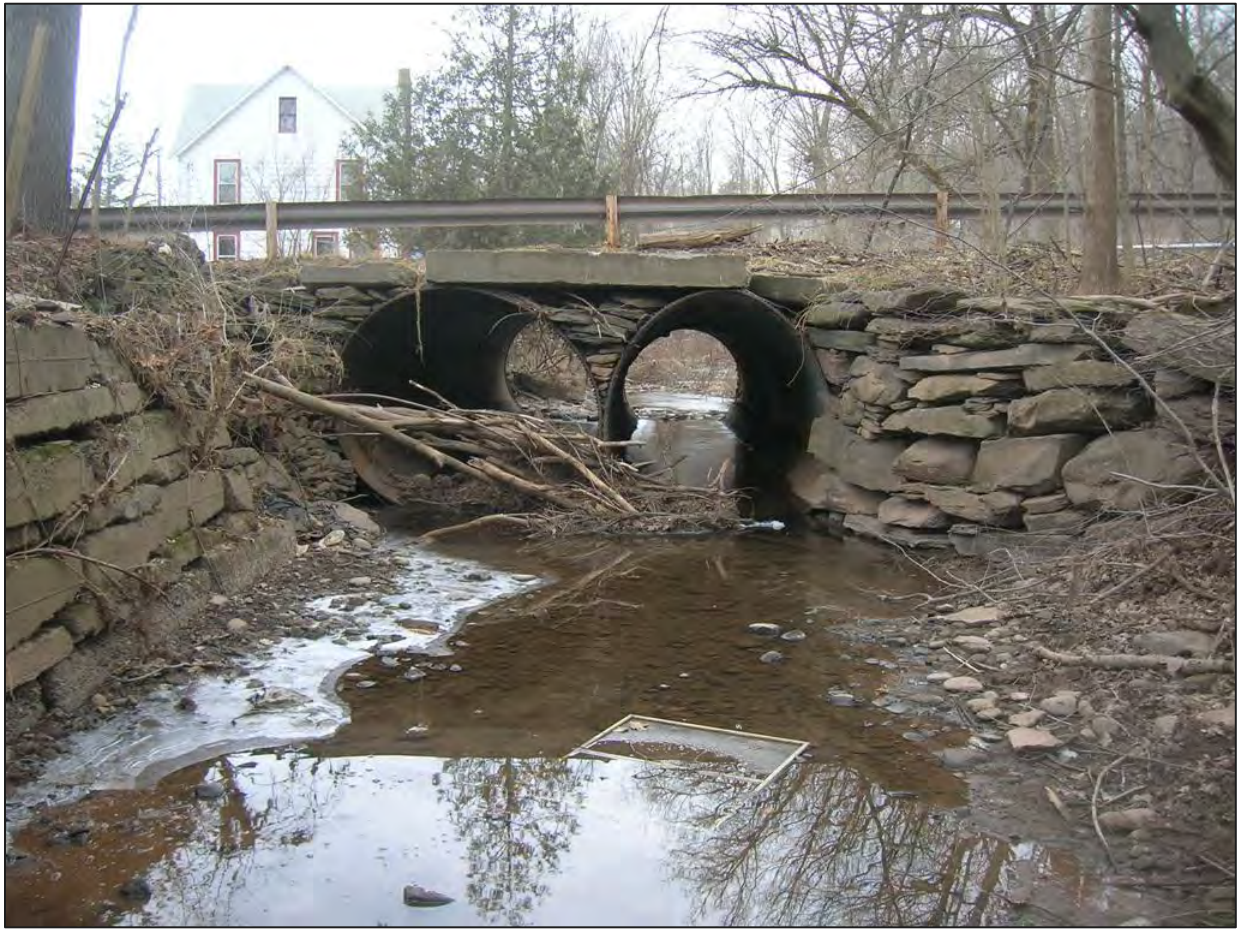
Figure 4-1: Inlet of Cemetery Road culvert, with debris in the channel
